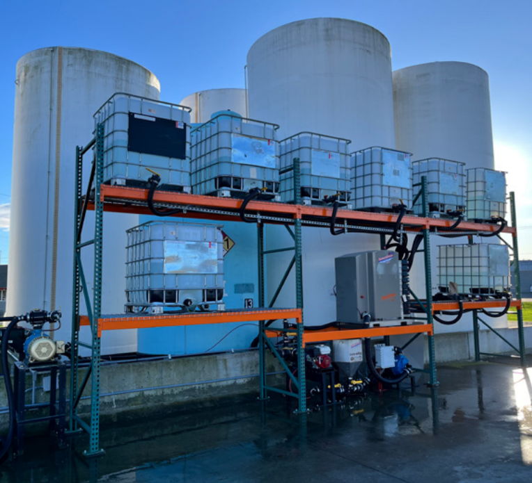
The SurePoint AG Quickdraw Automated Liquid Tender System recently installed at our Burlington Agronomy Plant. This system reduces mixing times up to 50% and can be run by one person.
